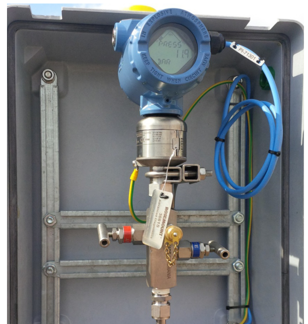
Rosemount 3051S installation
