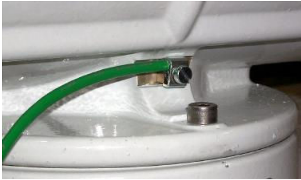
Figure 1-7: Ground Wire Removed
