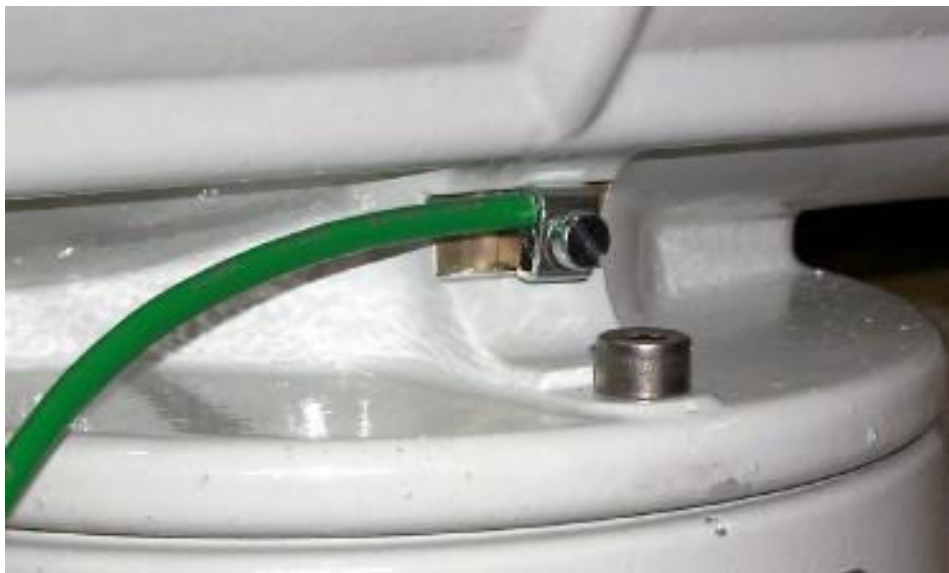
Figure 1-7: Ground Wire Removed
