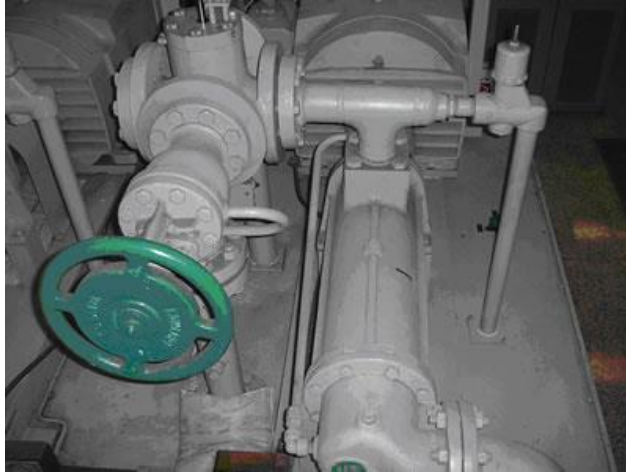
Figure 2. Solenoid – Operated Unloader (upper left) and Screw Pump (right)
