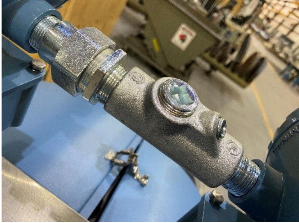
Figure 1-21: Explosion proof conduit screwed in each head
