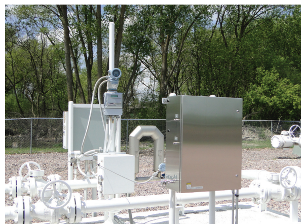
ELITE CMF Coriolis Meter installed with SGM and Sample Conditioning System
