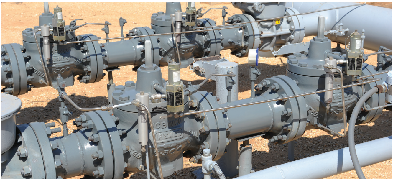
Figure 1. Natural Gas Distribution A typical dual run city gate station utilizes Type EZR's in a monitor configuration.
