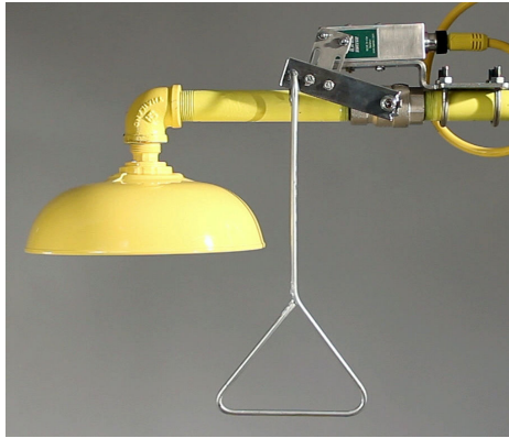
Figure 7-1: TopWorx Switch Installed on a Safety Shower
