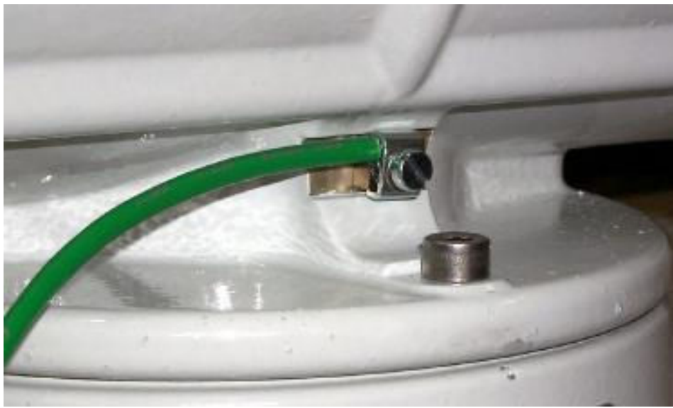
Figure 1-8: Ground Wire Removed
