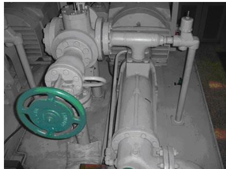
Solenoid – Operated Unloader (upper left) and Screw Pump (right)
