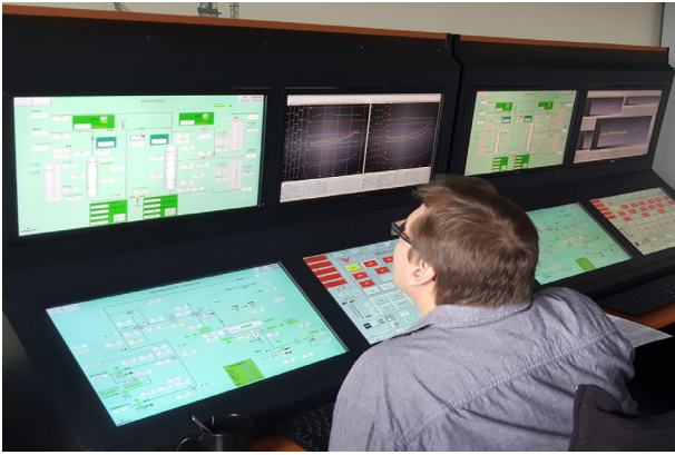
Figure 3. Using OTS enables operators to respond to process disturbances and upsets in a smoother way.
