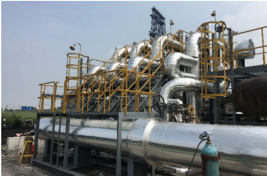
Figure 1. Mass and Watercut Metering System installed at refinery site in Tianjin.
