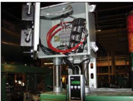
Compressed air flow meters are used on each case erector and flow is displayed and data-logged at a centralized location.
