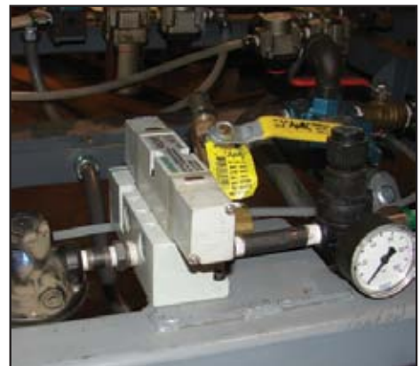
AFTER: The new 3-position Numatics valves reduced consumption to 15 cfm.
