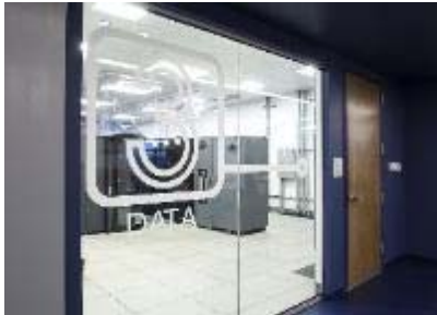
Data Center Thermal Management
